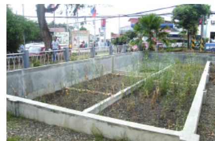
Figure 1: View of the aerobic treatment modules: planted gravel filter (PGF), indicator/polishing pond (IP). (Source: BORDA)
