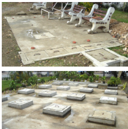
Figure 2: View of the anaerobic treatment modules: settling tank (ST), anaerobic baffled reactor (ABR) and anaerobic filter (AF). (Source: BORDA)
