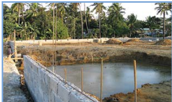
Construction of the first vertical flow treatment wetland for domestic waste in Bayawan City, Negros Oriental.
